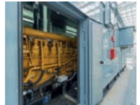
Top: light corridor Bottom: generator
